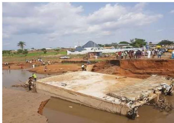
Figure 1.2: Alagbado bridge along Foma-river washed away by the flood.
